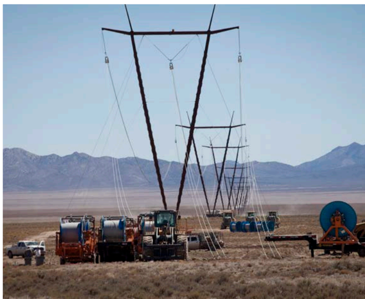
A VERY VORACIOUS VENTURE: Sturgeon Electric crews constructed 866 of these 146’ tubular guyed-V structures along the 235-mile route.
